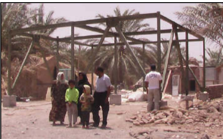
Family in front of the frame for their new shelter being constructed by RI
